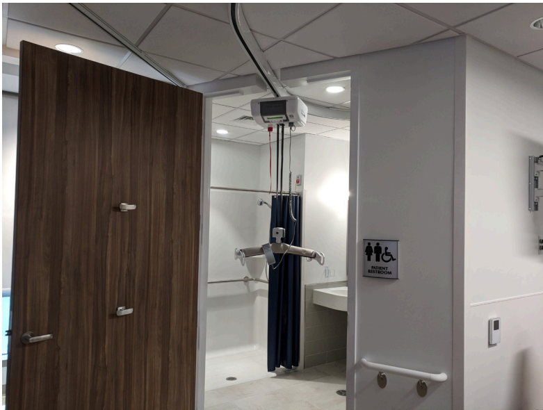
Full height doors can be specified to allow the track to pass into the bathroom.
