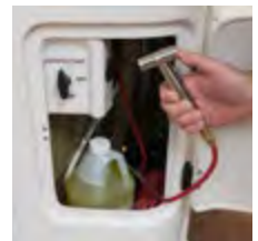
Built-in Disinfection System
